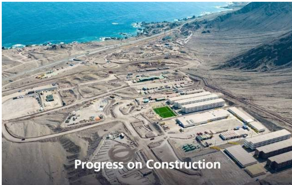
Photograph of Marubeni Corporation's desalination project for Codelco, in the Antofagasta Region.
